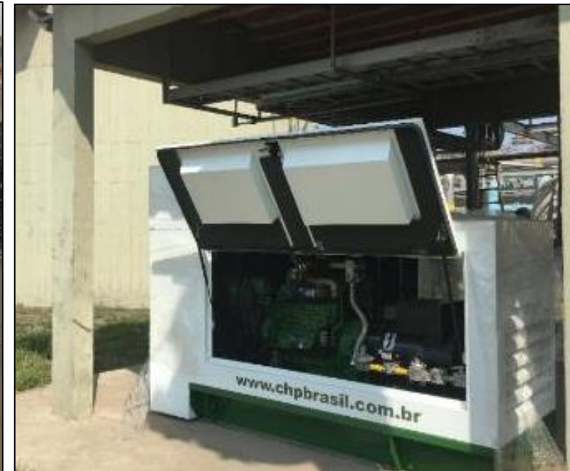
Biogas Electrical Use
