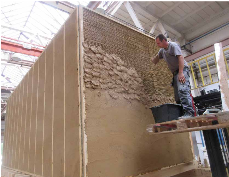
← Figure 4. The walls of the Zero Waste Space are made of sustainable building materials with good climatic qualities, including: wood, straw, flax fleece and clay. No additional plastic sheeting was used in the wall construction (Photo: Roland Meingast).
